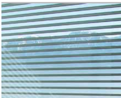
No visible vertical connections.
